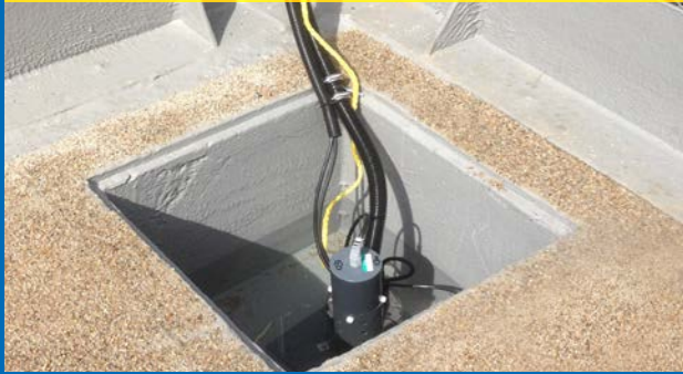
Sump Pump for Floor Voids under Timber Floors
